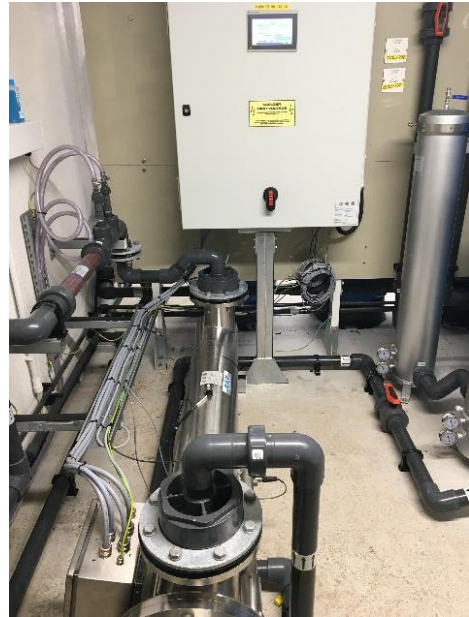
Fig 2 – Newly installed UV unit & system
